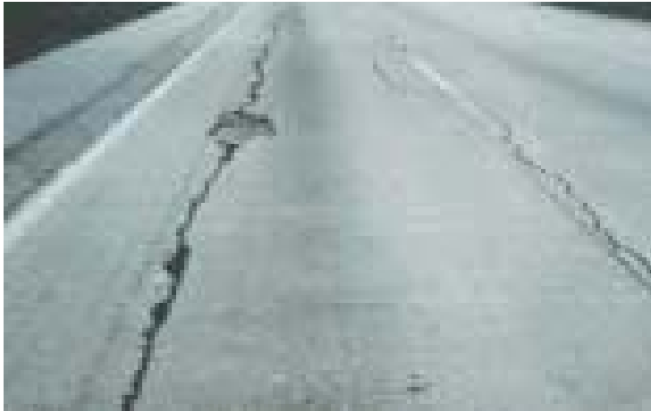
Figure 2.3 - Example of longitudinal cracks affecting condition rating on a roadway segment
