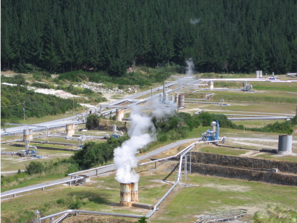
Figure 1.1 - Example Infrastructure Facility: A Geothermal Power Facility in New Zealand
