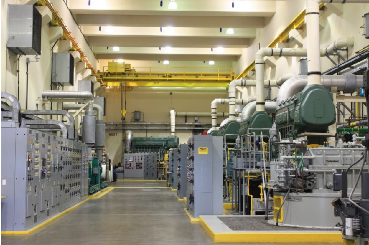
Figure 9.1 - Example of a Complex Machine Room
