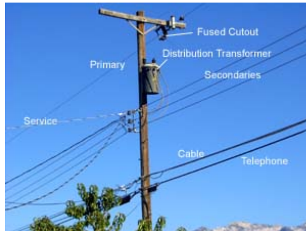
Figure 15.9 - Typical Residential Electricity Distribution Infrastructure
